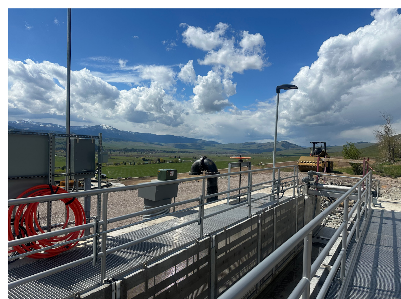
Modernized water delivery infrastructure within the Jocko Valley irrigation system.
